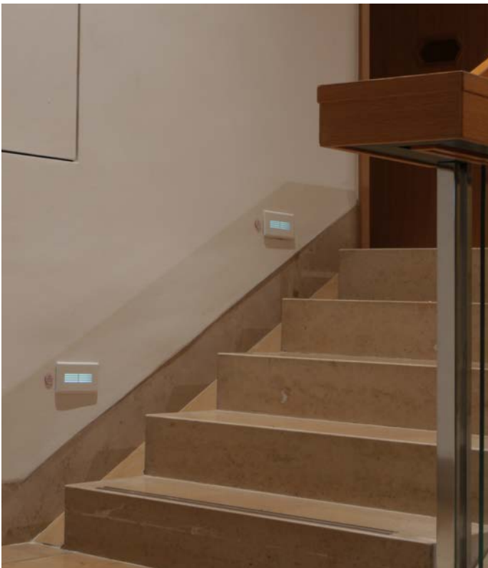
SN 6110 G LED step lights outside the auditorium
